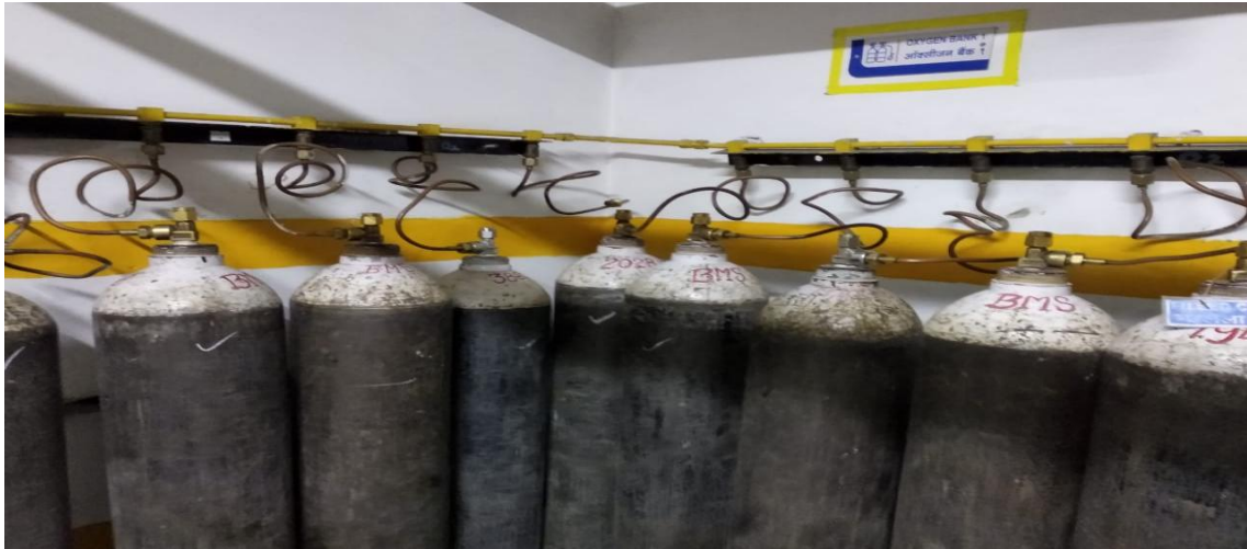
Fig. 2: Filled Oxygen Cylinder in Hospital with layout arrangement
